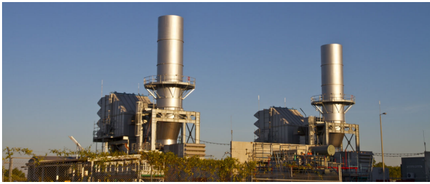
Figure 2: Combustion turbines that utilise high purity water injection
